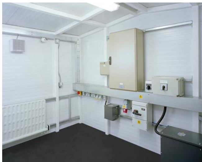
Internal view 4m x 4m instrument room
