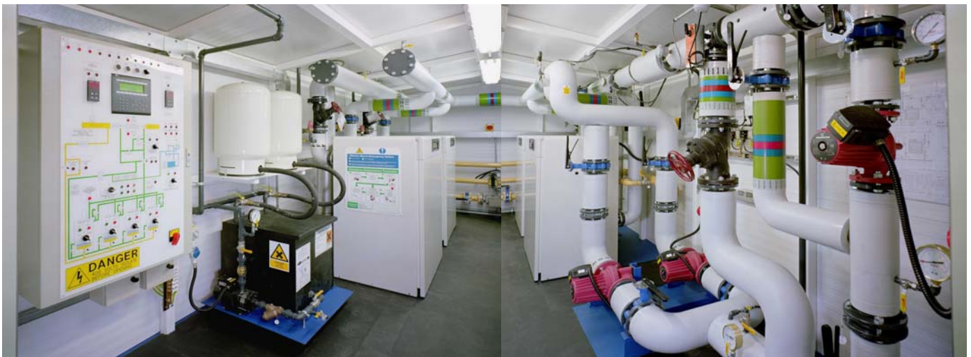
Internal View of 1MW Boiler House
